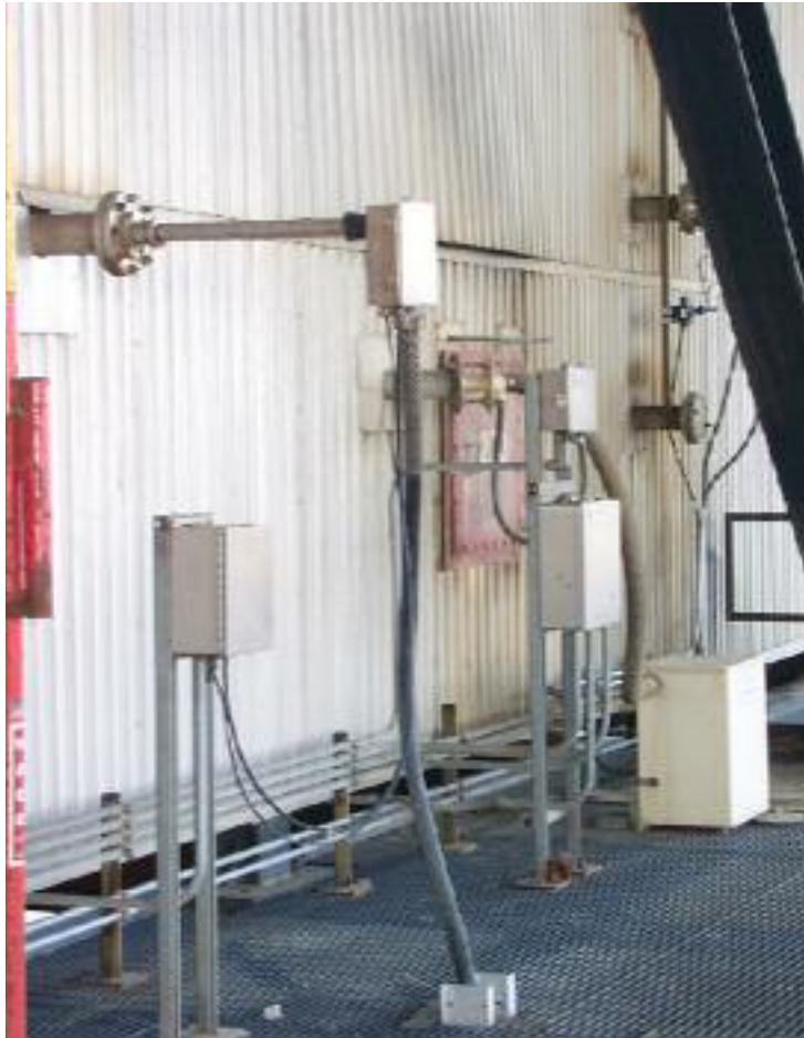
CEMS Probes In Outlet Duct
