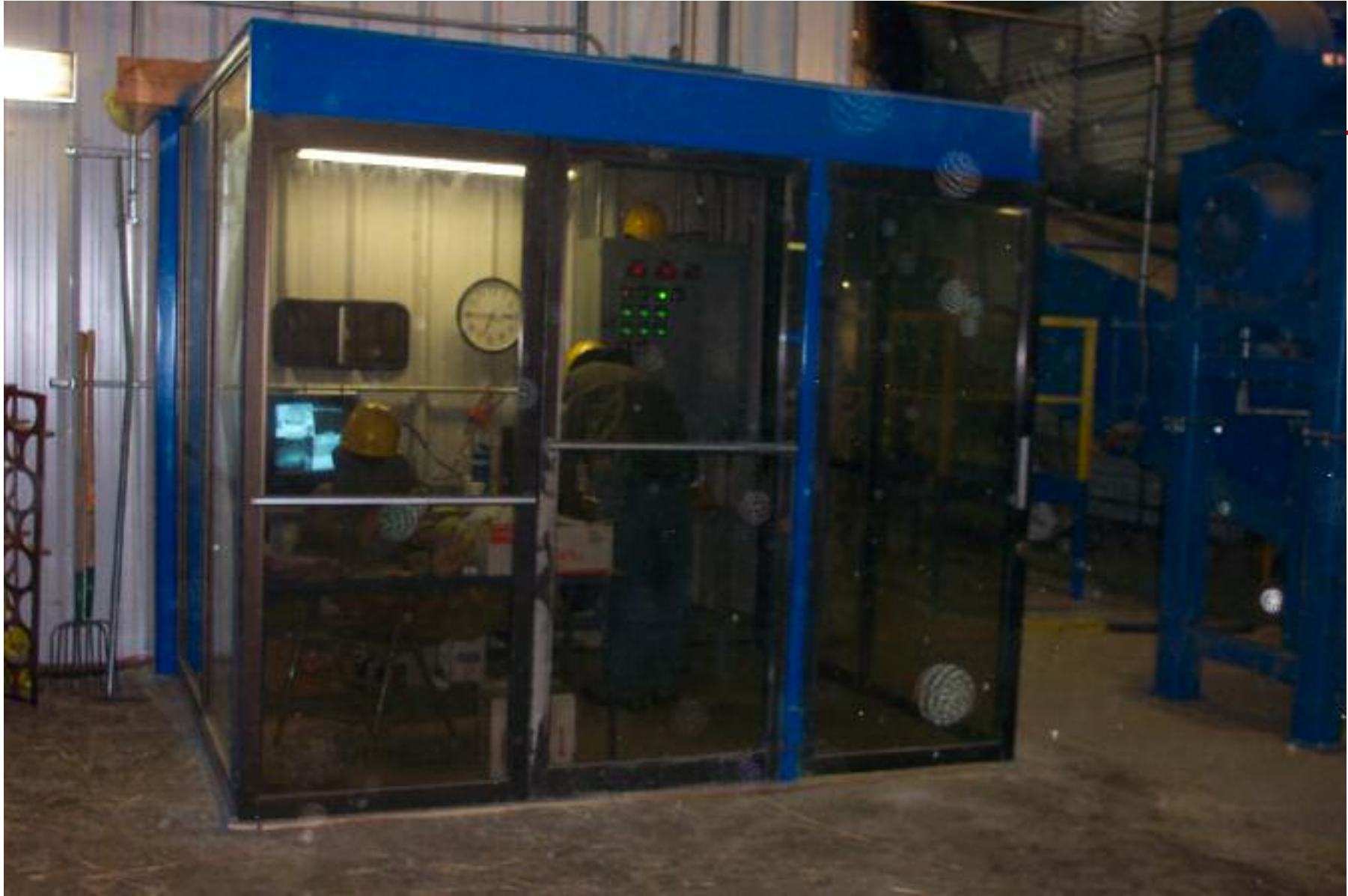
Switchgrass System Control Room.
