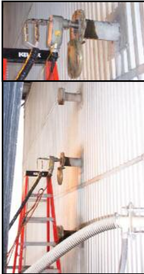
Emissions Probe In Outlet Duct
