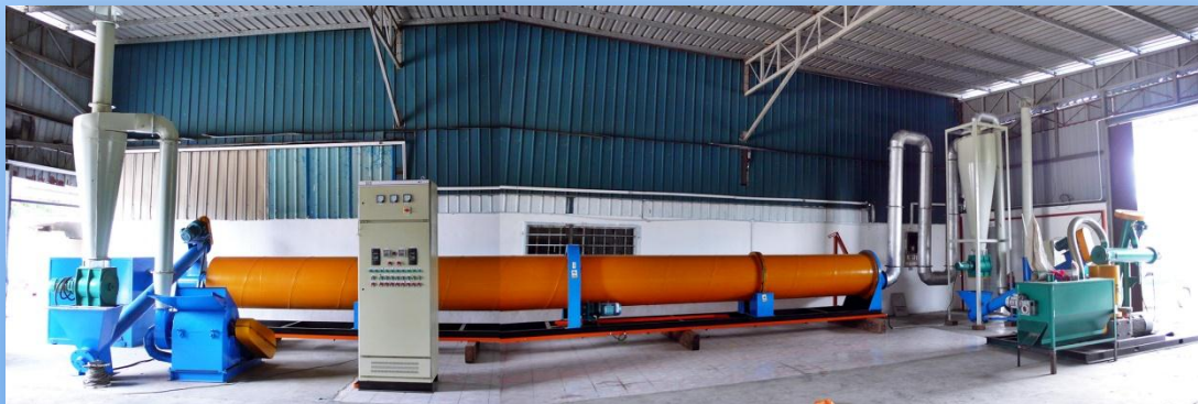
Biomass pelletising facility
