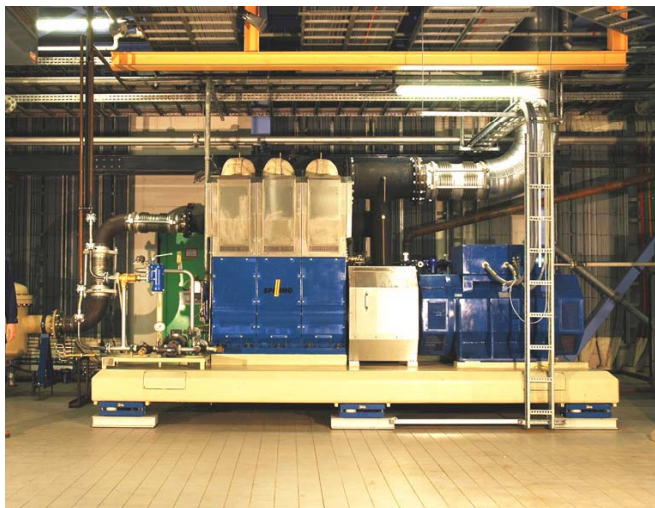
Bio Sludge Incineration Plant (Netherlands)
